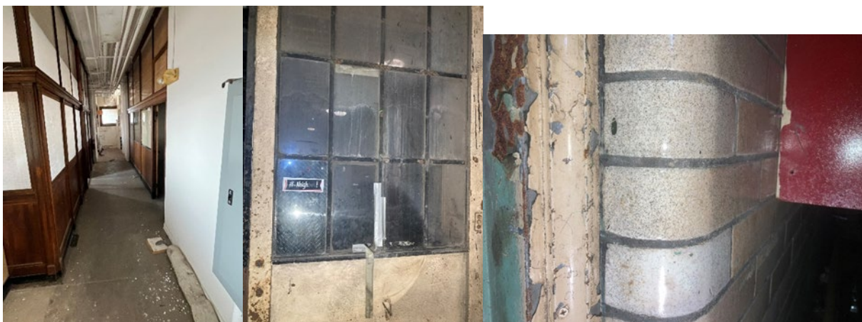
Figure 3-18. Examples of historic materials still extant on the building, include (left to right) wood paneling, metal windows, and enameled brick Source: Weston & Sampson site visit, 2024.
