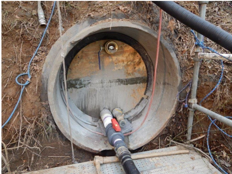
Photo from USACE Engineer Manual 1110-2-2902, Conduits, Pipes, and Culverts Associated with Dams and Levee Systems 16
