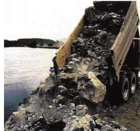
Figure D.10 Placement of Riprap. Careful use of an excavator may allow for more accurate placement than is shown above.
